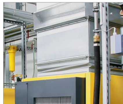
Fig. 2: Compressor ventilation connection with canvas duct joint
