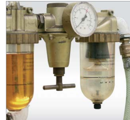
Fig. 6: Maintenance unit with pressure regulator
