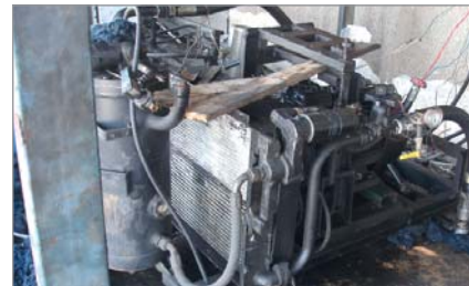
Fig. 1: Neglected compressed air station
